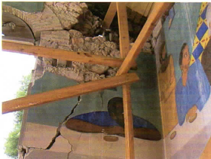
Detail of Philome Obin's damaged mural "The Last Supper" at Holy Trinity Cathedral. Conservation treatment to stabilize the mural is planned for fall 2010. Photograph by Stephanie Hornbeck
